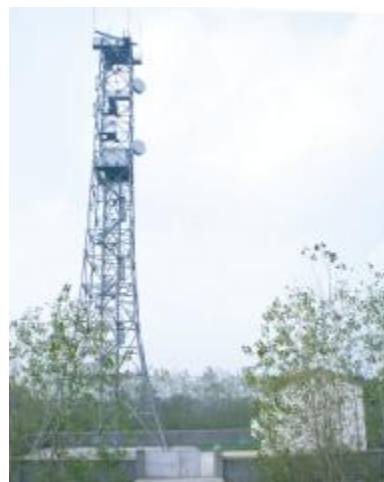
Fudewei radar station
